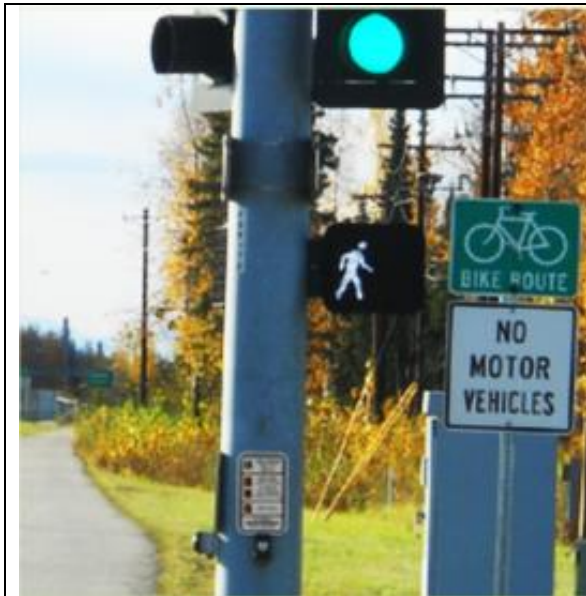
Signal with push button activator ii
